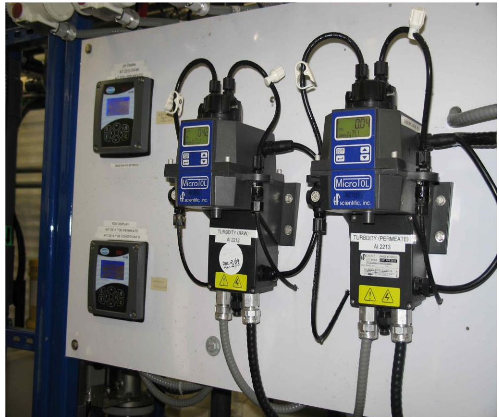
On-line turbidity meters
